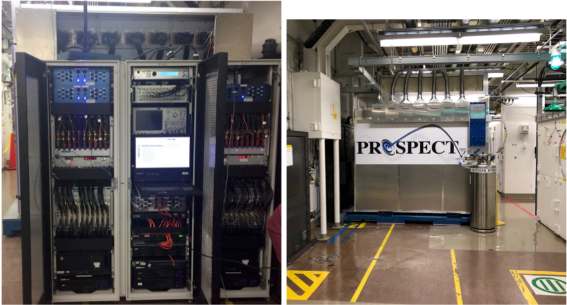
Figure 3.10: (left) Electronics racks and their contents during installation, before being mounted onto the outside of the shielding package. (right) View of full PROSPECT detector package from the West face. The calibration motor boxes are mounted to the side of the aluminum paneling, allowing radioactive sources to be transported through Teflon tubing from the top of each segment column. The slow-control panel (blue) is shown along with the liquid nitrogen dewar used for the boil off cover gas.
