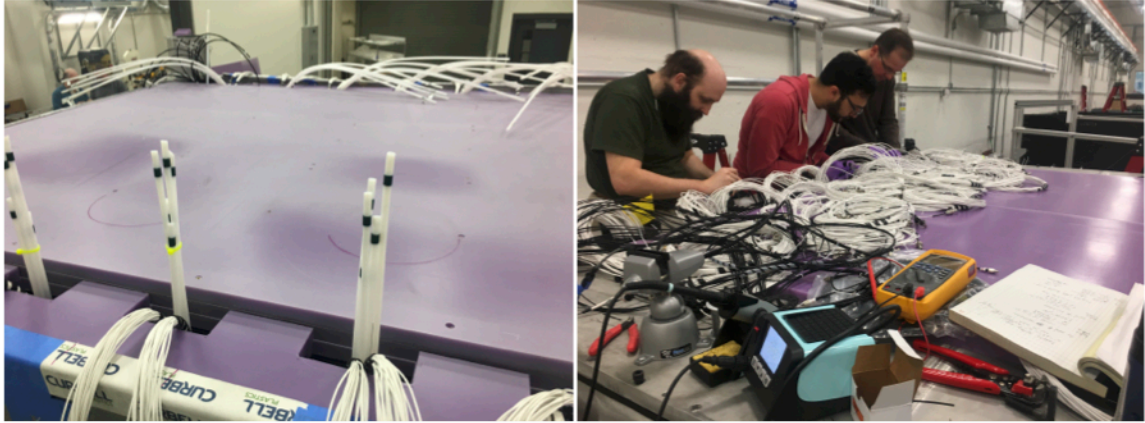
Figure 4.20: (left) Layers of BPE installed on top of the inner detector before the secondary tank lid is laid. Notches are cut into the edge pieces to allow for cabling and tubing to exit. (right) Collaborators helping to route cables through Icotek grommets. Equipment for the level sensor installation is also shown.
