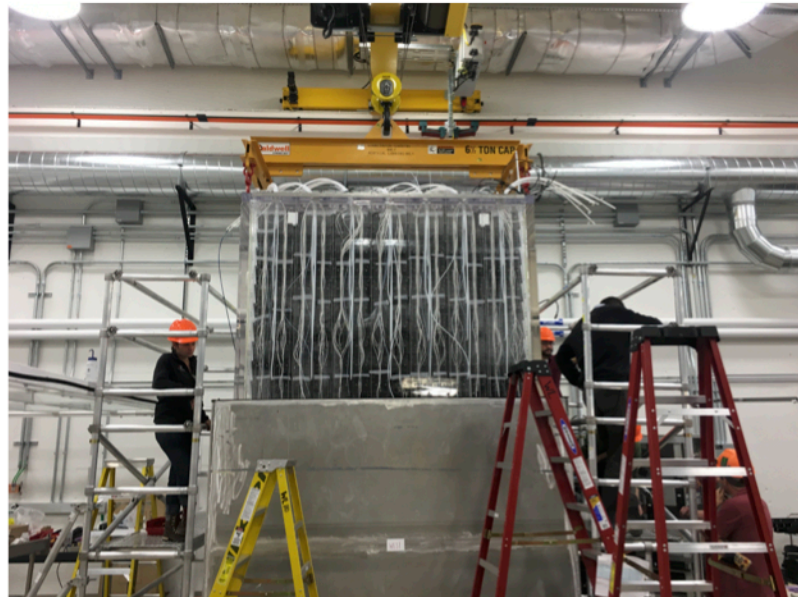
Figure 4.19: (top) Adding the acrylic tank lid after the inner detector was assembled and the acrylic side walls were installed. (bottom) The inner detector being lifted into secondary containment tank. Layers of BPE and plumbing lines were installed prior to the lift.
